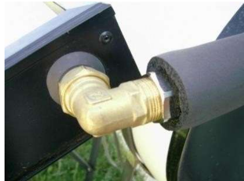
Photo – 2: Collector Upper-right tube connection
