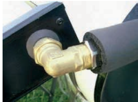
Photo – 2: Collector Upper-right tube connection
